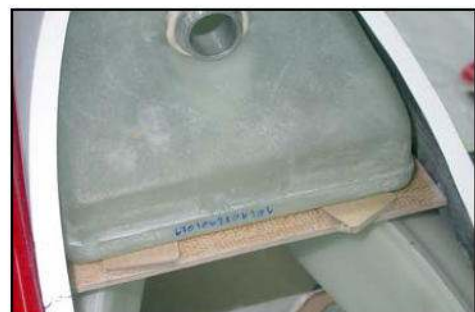
(below) Tack front front tank support in place with 3mm thick packers under the tank.
